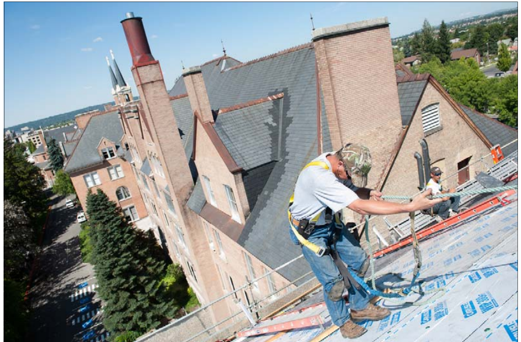
Workers spent the summer harnessed up – and ignoring the great views from the roof of College Hall.
