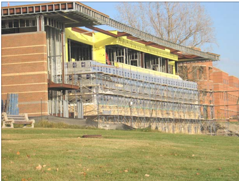
PACCAR Center for Applied Science is rising fast just south of the Herak Engineering Building. Huffman Contractors' crew will focus on interior work with the onset of cold weather.
