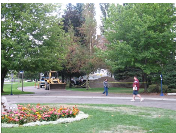
The sizeable piles of sand seen in front of the Admin Building at the start of the semester were due to removal of rubble and concrete that filled in the old, basement-level swimming pool.
