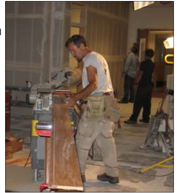
Chris Czech of Walker Construction works on renovation of the Admin Building lower level.
