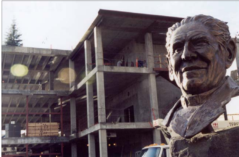
Father Art Dussault, S.J., is considered the master architect of Gonzaga's landscape, and he is still watching over campus construction, 12 years after his death.
